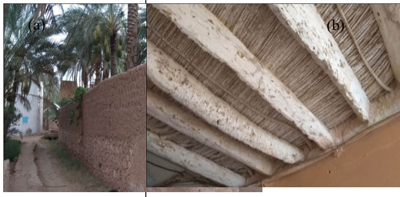
Fig.10: (a) adobe wall; (b) Stone vault with Timchent and trunks of palm in Béni Isguen
